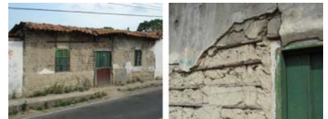
Figure 16. Low adherence of plaster due to weathering effects and missing connection to the wall materials
