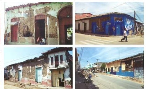
Figure 19. Structural damage to bahareque dwellings in the city of San Vicente caused by the earthquake on February 13, 2001.
