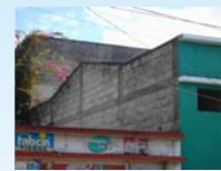
Figure 13. CBrc - Confined concrete blocks
