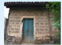
Figure 14. Pdc - 'Piedra de Canter' masonry of cut quarry stones, confined with timber elements
