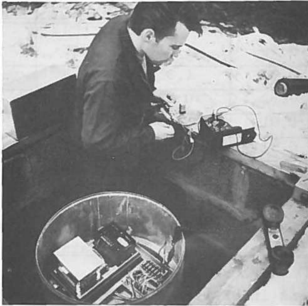
Figure 4.3 Technician adjusting damping resistor at the WHV.
