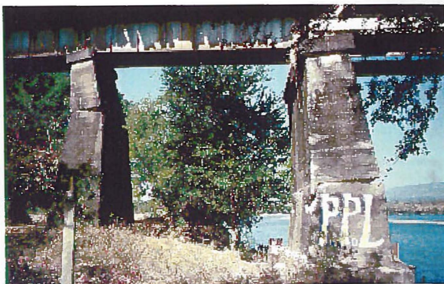
Virkinger av jordskjelvet i El Salvador 13. januar 2001 (M=7.6). Bildet viser en jernbanebro. Effects of the El Salvador earthquake 13 January 2001 (M=7.6). The picture shows broken piers of an old railway bridge.
