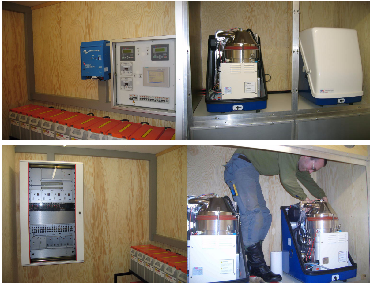
Fig. 4.4.5. The figure shows, in the upper left part, the battery bank and the unit for controlling battery charging and control of the Stirling generators. In the lower left part, the array concentrator rack is displayed. The upper and lower right hand parts show the two Stirling generators. The windmill is the primary source for charging the batteries. The control unit measures battery charge, room temperature and the temperature of the 1000 liters water tank. A programmable algorithm in the control unit will start and stop the generators as needed. The generators can also be controlled by the use of a GSM phone. Remote access through the network to the control unit will be installed later.
