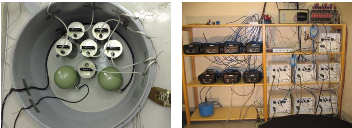
Figure 6.5.1. Left: One of the three pits in the Long-Period Vault (LPV) of the NOA subarray NC6. Right: Shelf with data acquisition equipment.
