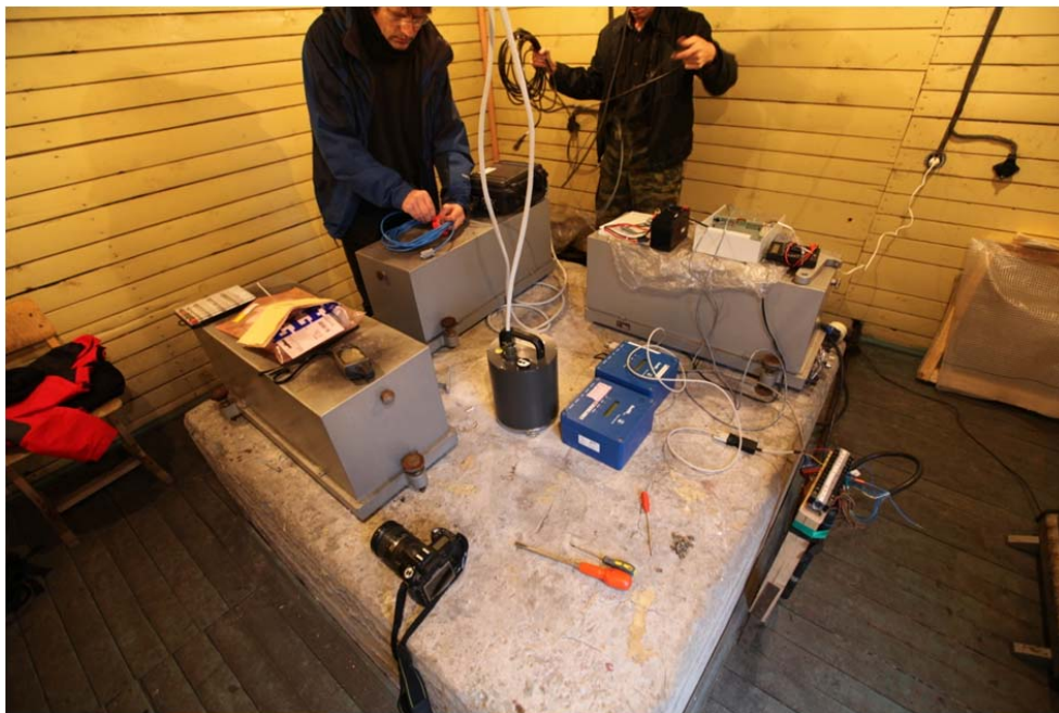
Fig. 6.3.5. Inside the BRBA site. The broadband sensor in the middle of the concrete pillar (dark grey cylinder) is replacing the three obsolete analog short-period Kirnos sensors (grey covers) and the experimental short-period GeoSig systems (blue boxes).
