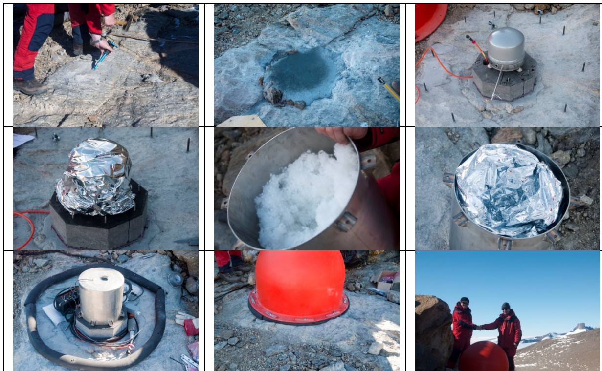
Fig. 6.2.3 Pictures from building the new seismometer station TROLL (progress from top to bottom and left to right): Flattening the bedrock surface; making a small fundement of cement; placing the oriented seismometer on a granite base; packing the seismometer in a first-aid-sheet for temperature protection; filling a steel casing with insulation material and placing it over the seismometer to avoid thermal convection of the air around the seismometer and protect it against rapid air pressure changes; installing cables, digitizer and GPS antenna; covering the whole with a double walled plastic dome, which is screwed to the bedrock; work done.
