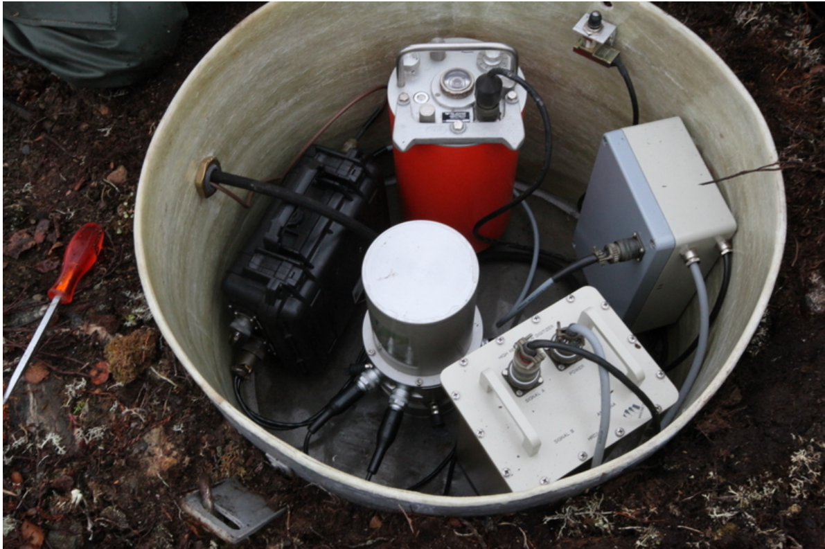
Fig. 6.4.1 ARCES seismic and infrasound instrumentation, as installed in the field.
