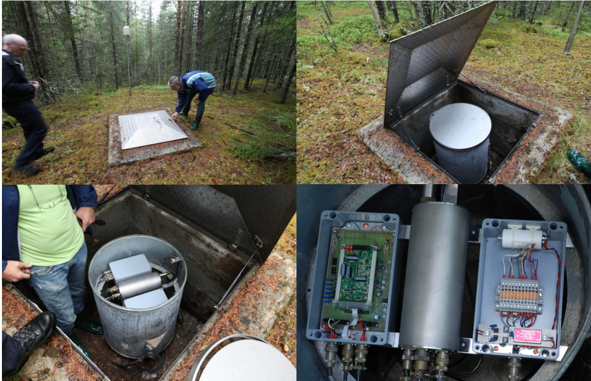
Fig. 6.2.4. Borehole site (BS) NC601. The sensor is installed in a shallow (down to 12 m depth) borehole. A zinc drum on top of the borehole contains the digitizer (Güralp CMG-DM24S3EAM), a power and communication pit box (lightning protection, battery power charger, Patton modem, 12V 800mAh battery bank) and a junction box (coarse lightning protection and 48/12 DC/DC converter).
