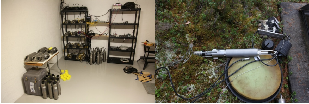
Fig. 6.2.7. Güralp CMG-3V Hybrid borehole sensors. Left: Test setup, right: just before installation with hole lock attached.
