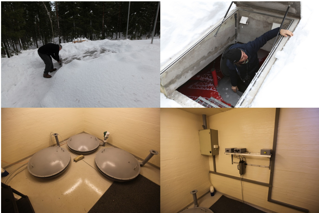
Fig. 6.2.3. Vault site (VS) at NC6. The VSs have 3 pits (formerly used for the 3 components of long-period sensors). With the current installation only one of the pits is used.
