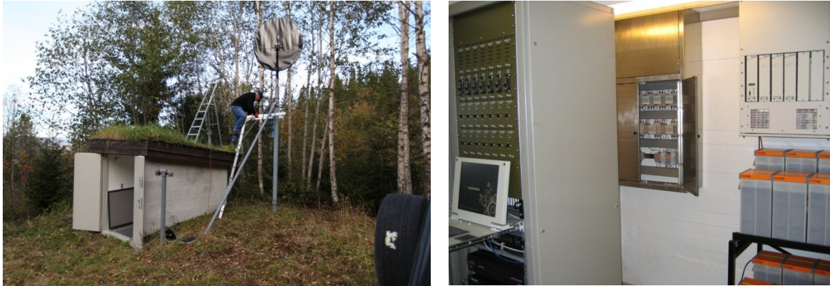
Fig. 6.2.2. Central Terminal Vault (CVT) at NAO. In 2012 NORSAR migrated to new VSAT technology and the antenna dish needed to be pointed to a new satellite. Right: Inside of the CVT. From left to right: rack with modems and power distribution to pits, cable box to pits with coarse lightning protection, and uninterruptable power system with battery rack.
