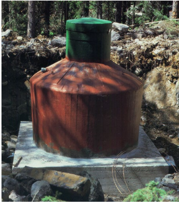
Fig 5.1.3 The seismometers and associated electronics of NORESS were placed on concrete pads and housed inside fiberglass tanks.
